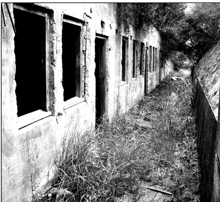
WWII munitions railway in disrepair (all photos: Peter Ryan)
